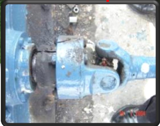
Coupling Long Shaft Pecah
